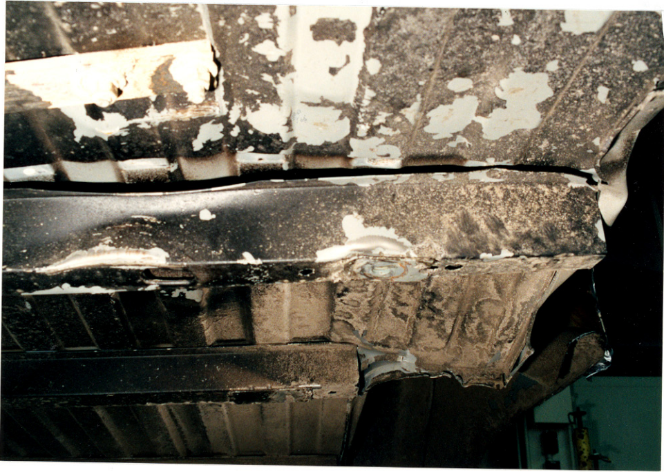
17. Close-up view of the cargo bed looking from front to back along the left side in the area over the failed CNG tank
